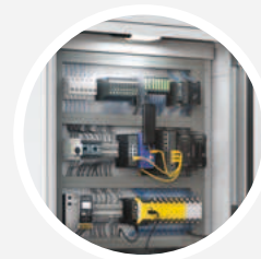
Control panel technology, DIN rail terminal blocks
